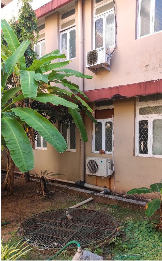
Rainwater Harvesting Sytem
