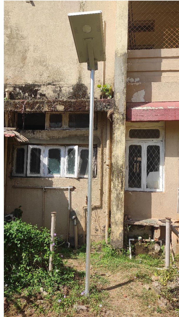
External LED Solar Lights
